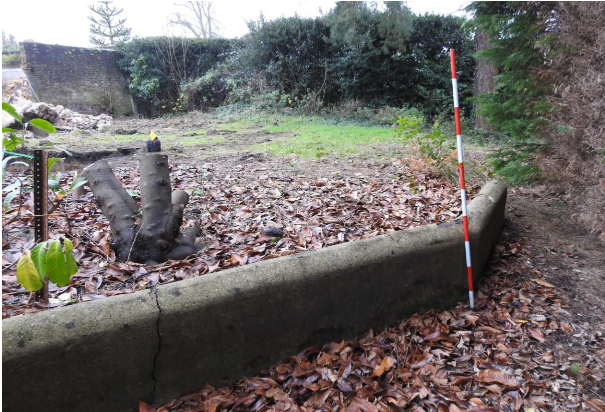
Plate 7: Showing retention wall containing vast levelling deposit exposed in Evaluation Trench 2. Looking south-east with two-metre scale.
