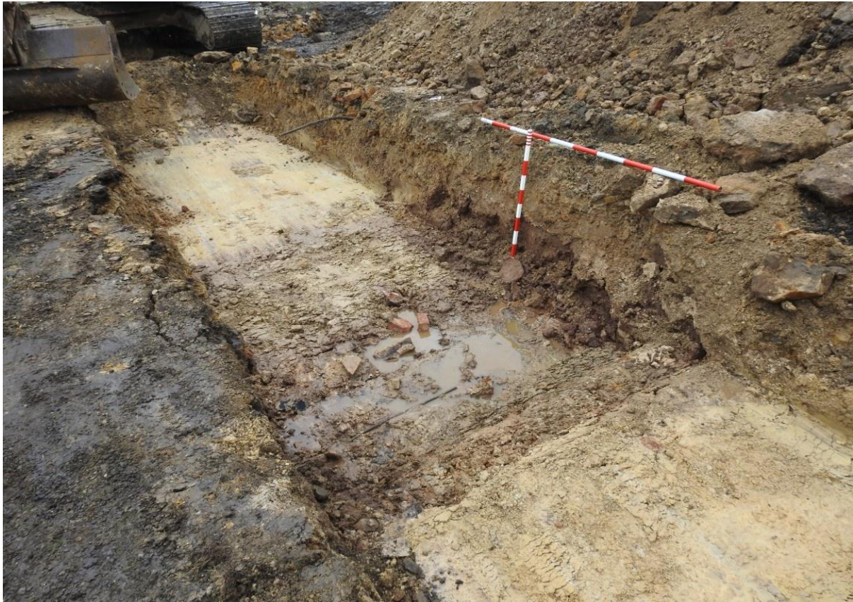
Plate 9: Showing exposed construction cut or collapsed manhole/ drainage duct [303]. Looking north with one- and two-metre scales.
