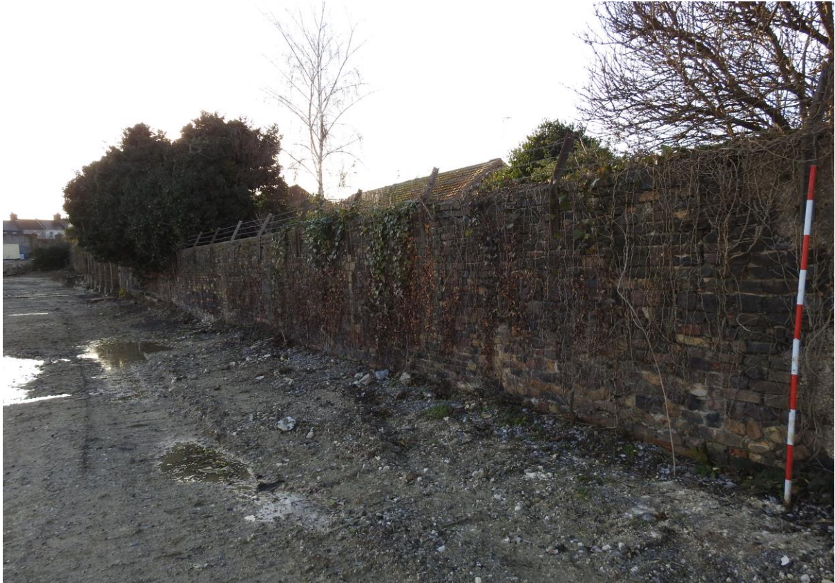
Plate 33: Northern section of north-western boundary wall. Point Z1 in background. Looking south-west with two-metre scale.
