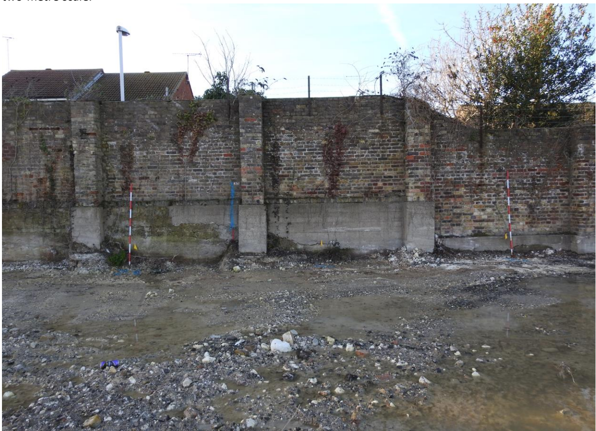
Plate 34: Showing Section Z1-Z3 at southern part of western boundary wall. Looking west with two-metre scales.
