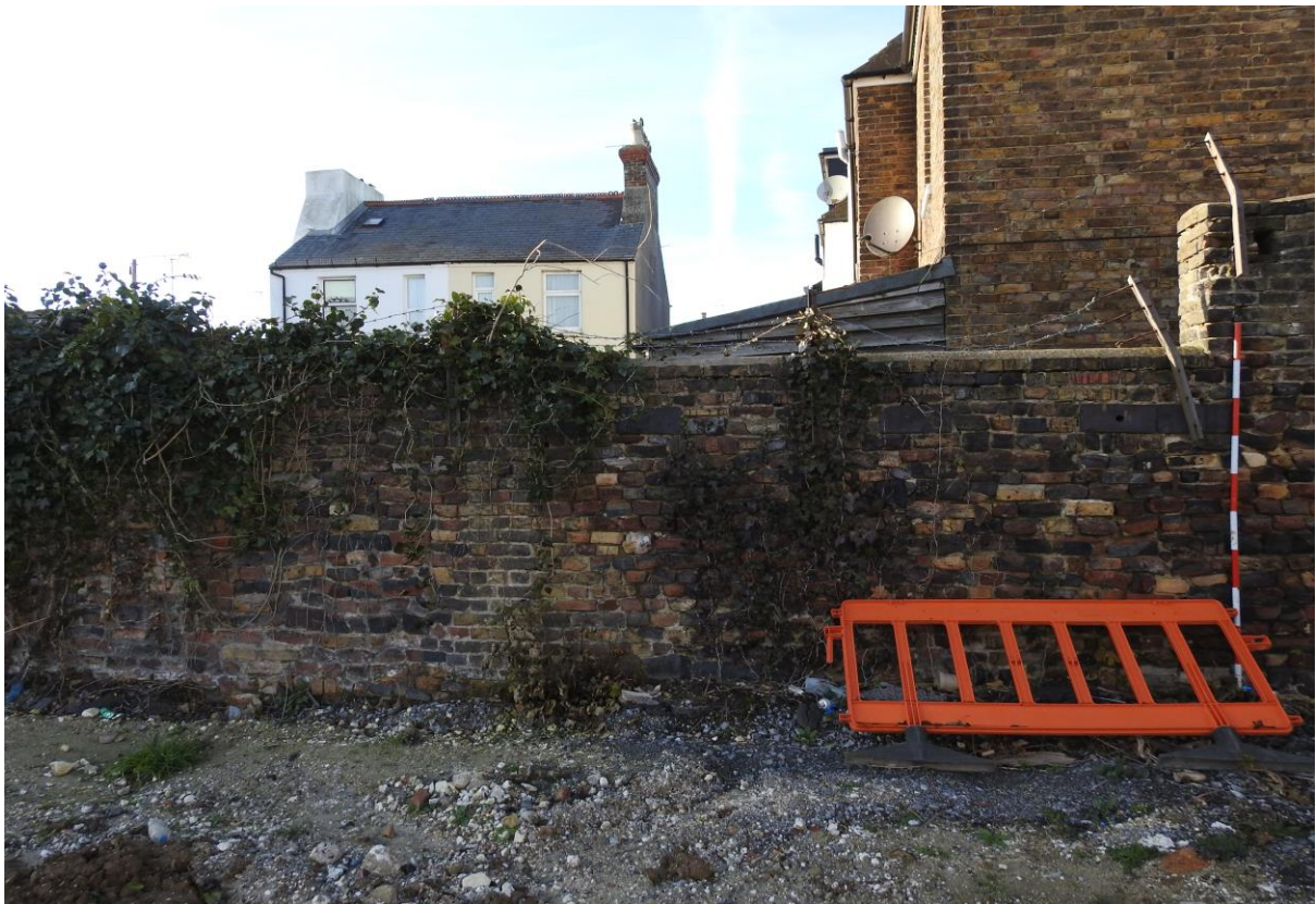
Plate 32: Showing section of north-western wall (approx. 6 metres) at northern corner of the Site. Looking north-west with two-metre scale.
