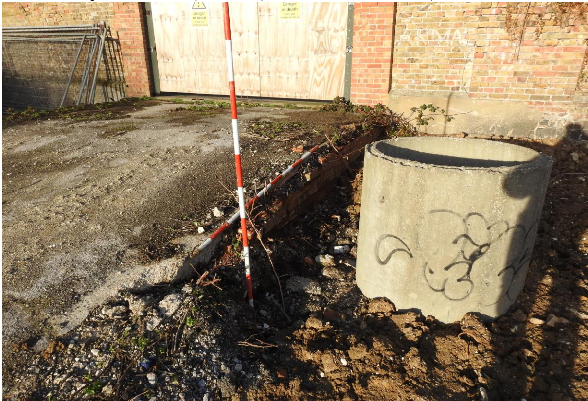
Plate 30: Showing exposed ramp at northern gate (adjacent to northern corner of PDA). Looking north with two-metre scales.
