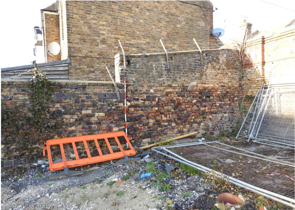
Plate 31: Showing section of north-western wall (approx. 8 metres) at northern corner of the Site. Looking north-west with two-metre scales.
