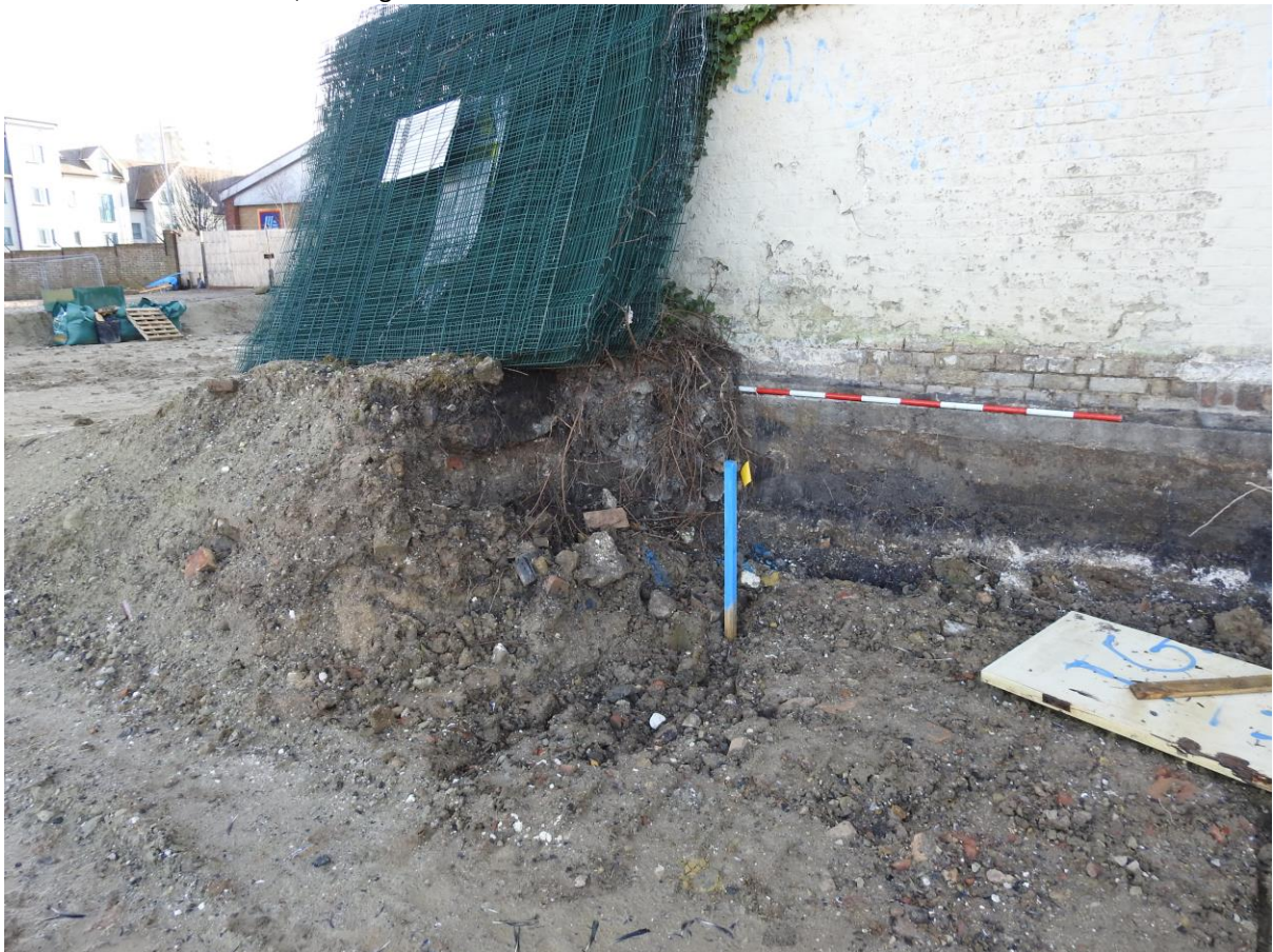
Plate 12: Showing loose loam with rubble forming batter that extends from X11 to south-eastern gate which is visible in background. Looking south-east with two-metre scale.
